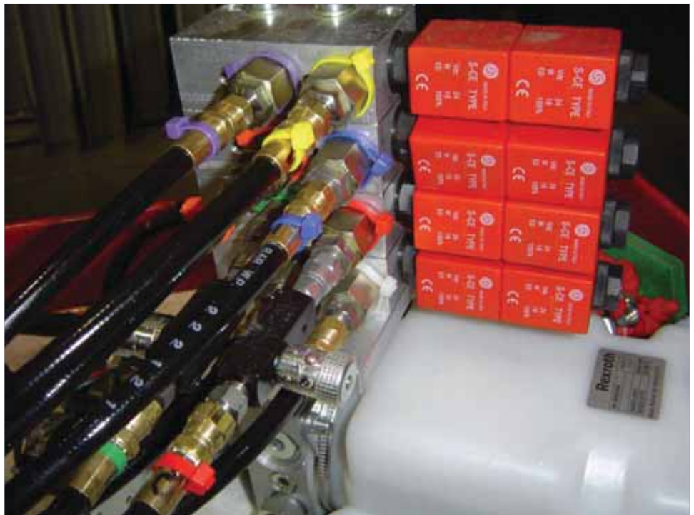
Figure 5c: Color Coded Hoses on Manifold
