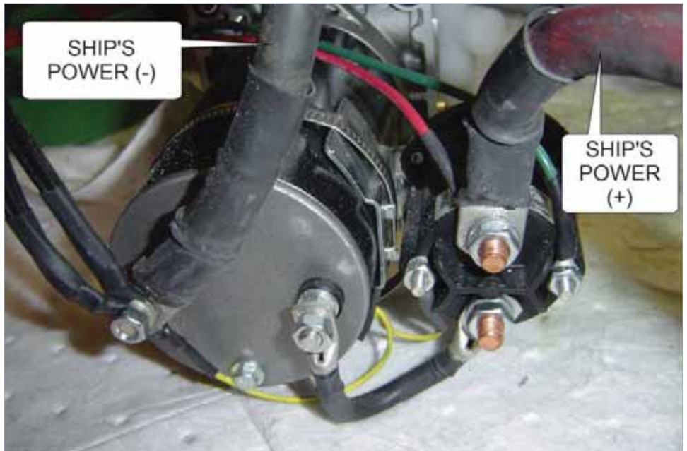
Figure 5b: Pump Motor Solenoid Wiring
